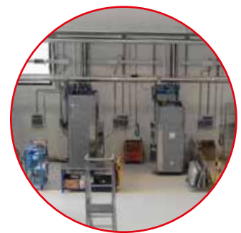
Lean Assembly stations for internal commissioning and FATs
