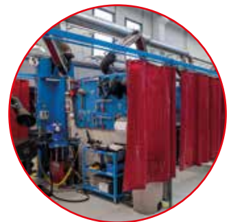
Manual welding stations for certified operators
